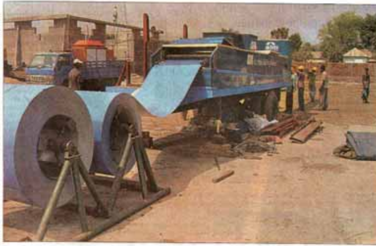
Steel coil is being shaped in line with the customer requirements at a construction site. ALM Steel Building Technology Ltd has brought in Automatic Building Machine technology to construct an infrastructure within a short span with a small manpower and lower costs.
